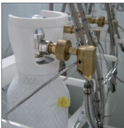
High pressure hose connected to the cylinder
